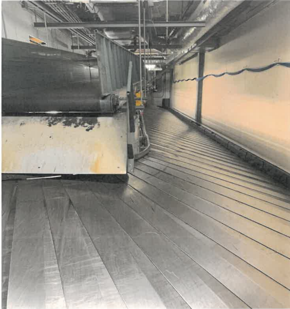
Incoming Baggage Belt, Baggage drop off
